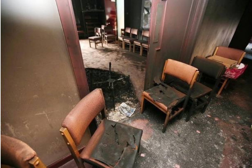
Arson attack on Cairns Hill Methodist Church in south Belfast leaves severe damage to the building. Picture by Jonathan Porter/PressEye
